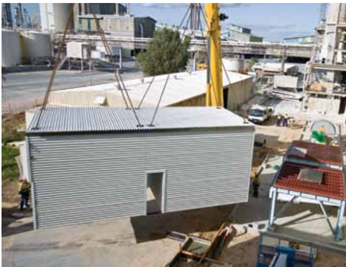
Left: The regenerative thermal oxidiser unit being lifted into position at WesCEF's fertiliser operations in Kwinana, Western Australia.
