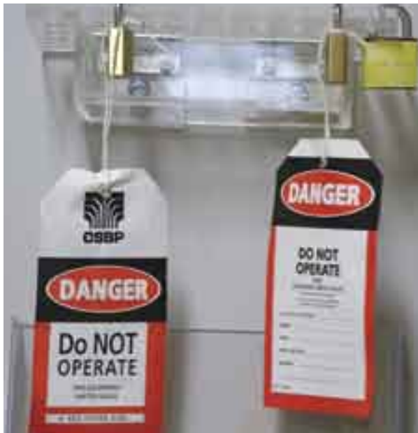
A new permit to work system has been introduced which includes the use of locks.
