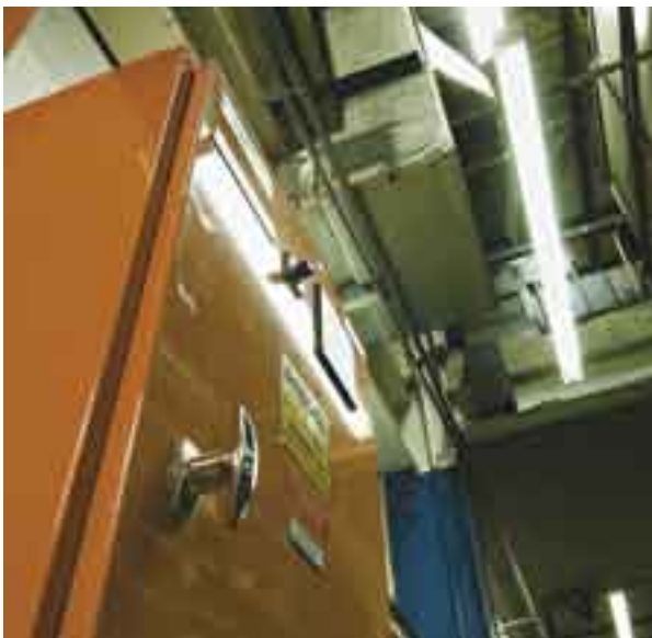
Power factor unit at Bakers Construction and Industrial, Blacktown, New South Wales.
