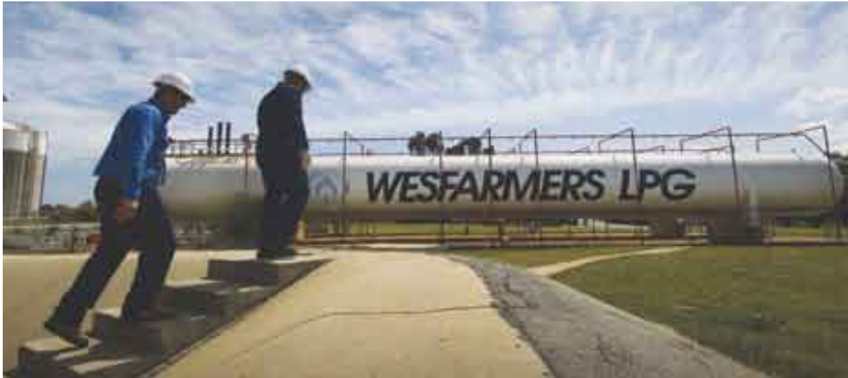
The LPG domestic storage tank at Kwinana.
