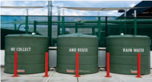
Rainwater collection tanks outside the Bunnings Box Hill warehouse, Victoria.
