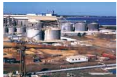
Demolition of the 92 metre stack at the sulphuric acid plant at Kwinana.
