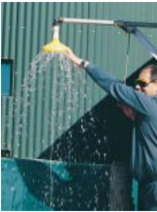
Above Testing a chemical shower near the chemical storage tank at Mundijong.
