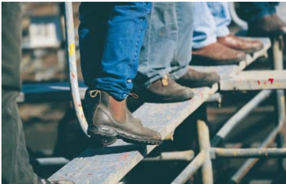
Above Wesfarmers Dalgety's saleyards at Boyanup, WA, showing walkways treated with non-slip paint.
