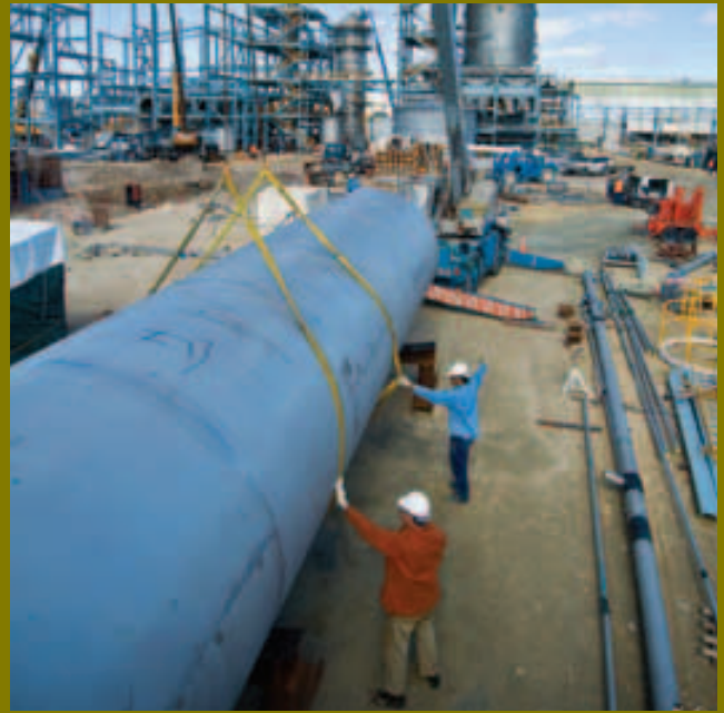
Work continued during the year on the construction of the new ammonium nitrate facilities, at Kwinana, Western Australia.
